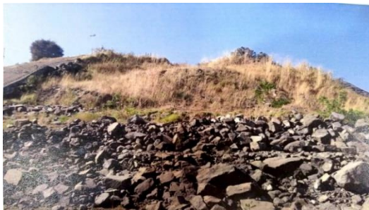
Fig. 3. Divide bund after distress
