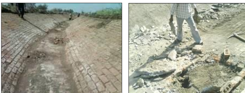
Photographs 1 and 2. Swelling of bed and sides and pipings from sides of Canal
