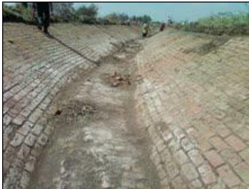
Photograph 12. Swelling of bed and sides of canal
