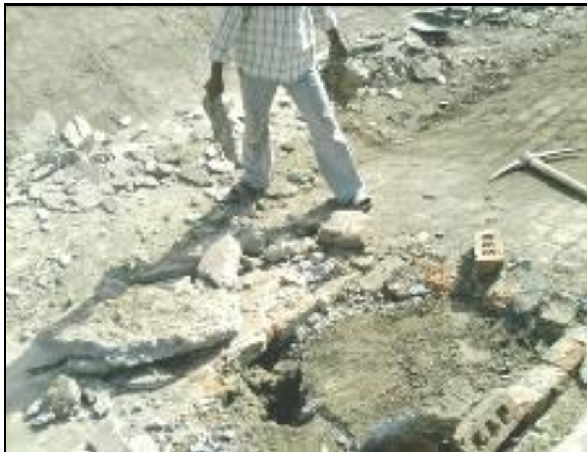
Photograph 14. Piping from sides of the canal
