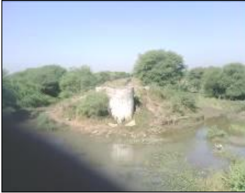
Photograph 13. Leakage from canal
