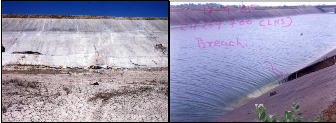
Photograph 1 and Photograph 2. Defects in lining and breach in initial stage
