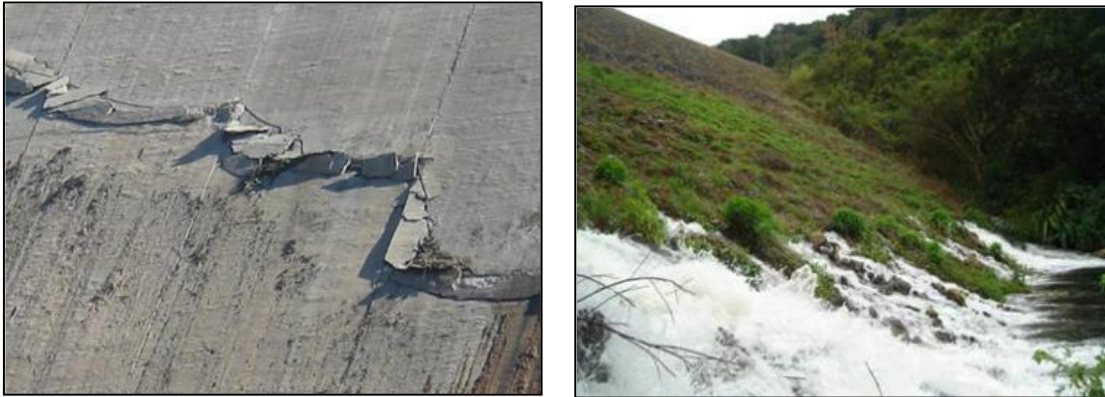
Figure 4 and 5. Damage to a Concrete Facing due to Rockfill Deformations (left) and Large Water Loss Crossing the Embankment, Consequence of Invisible Damages to the Facing (right).
